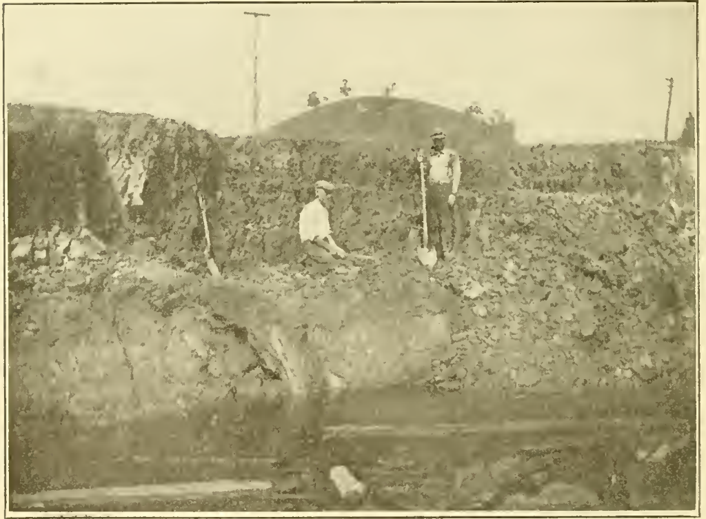
FIG. 2. Near view of the cave-in at "Well No. 69."
