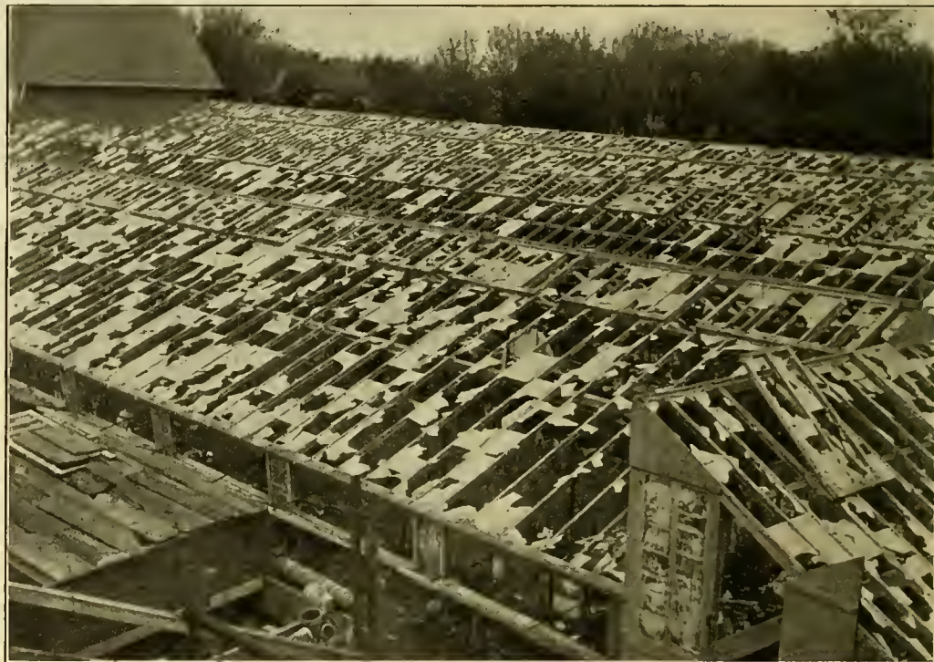
EFFECTS OF HAIL STORM, MAY 8, 1905, AT ESTABLISHMENT OF JOHN STAMM, HUTCHINSON, KAN.
