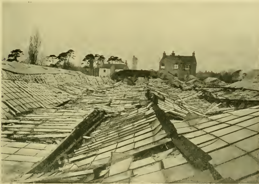
FIG. 72.—PLANT HOUSES DESTROYED BY SNOW IN A MARKET NURSERY.
