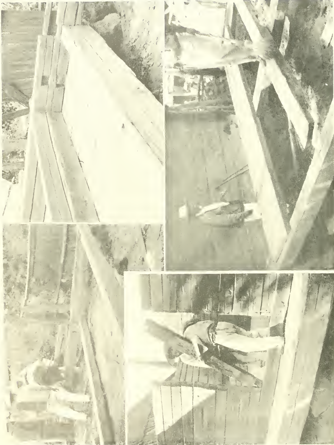
Upper (left): Leveling the foundation beams for a house. Upper (right): The "planchas" in position. Two side wall planks and one front wall plank in place. Notice the mortice for a pillar in the front "plancha." Lower (left): Placing one of the doorframes. Lower (right): Laying the floor boards of a house.
