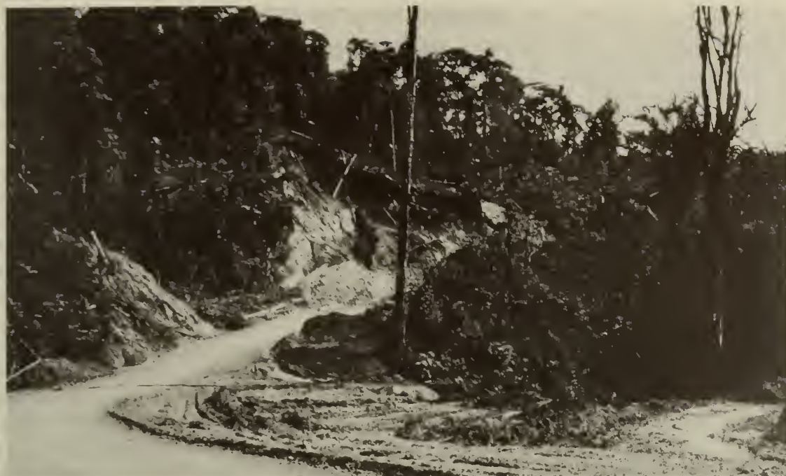
Figure 18: Road construction near Rincón. Note the erosion of the road cut exposing the red latosol soil. Photographed in February, 1985.
