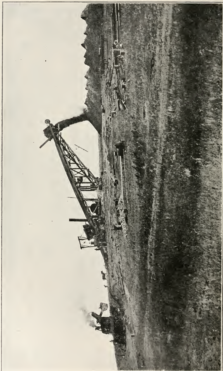
Steam Shovel and Derrick Cars in Operation on Big Cut at Station 300 on Inlet Canal, Belle Fourche Project, S. D.
