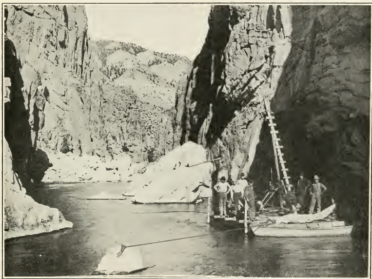
Diamond Drill on Barge in Shoshone River at Dam Site, Shoshone Project, Wyoming
