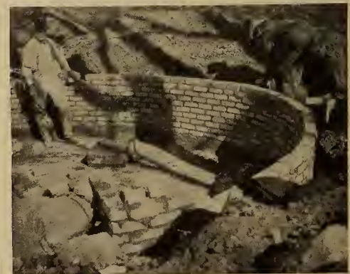
A single brick wall served as a frame for the concrete walls of the pond
