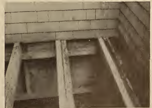
These piazza supports rotted and weakened the flooring. Part of it was removed and 2-inch planks were nailed to the old stringers
