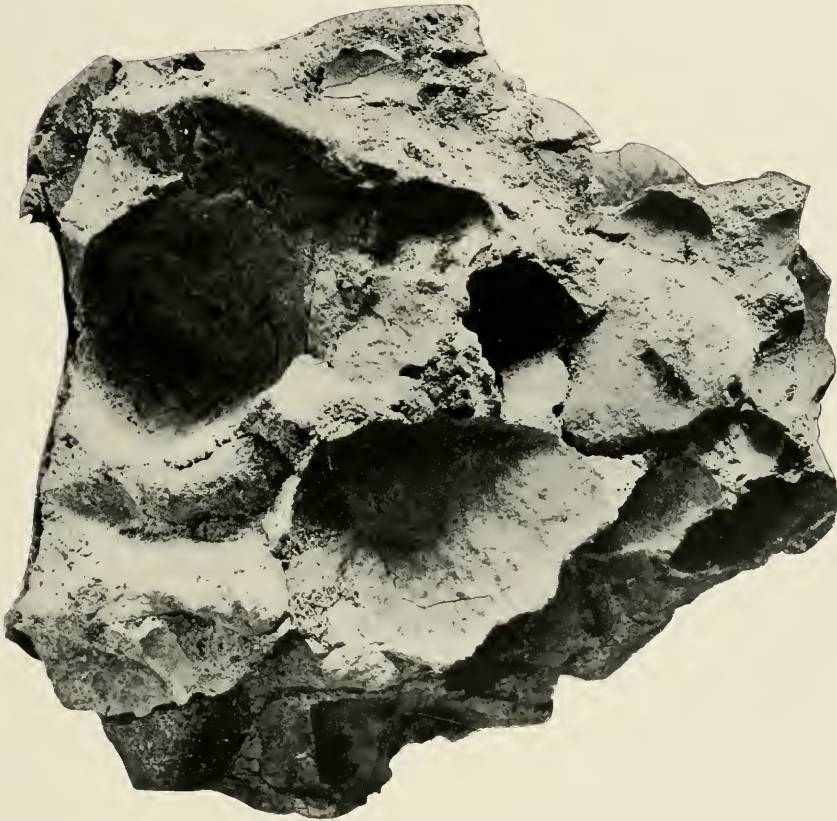
PLATE L. CONE FROM CRUSHED CUBE OF CONCRETE FROM ABATAN RIVER, CORTES, BOHOL, SHOWING EFFECT OF USING GRAVEL COVERED WITH GREEN ALGÆ.
