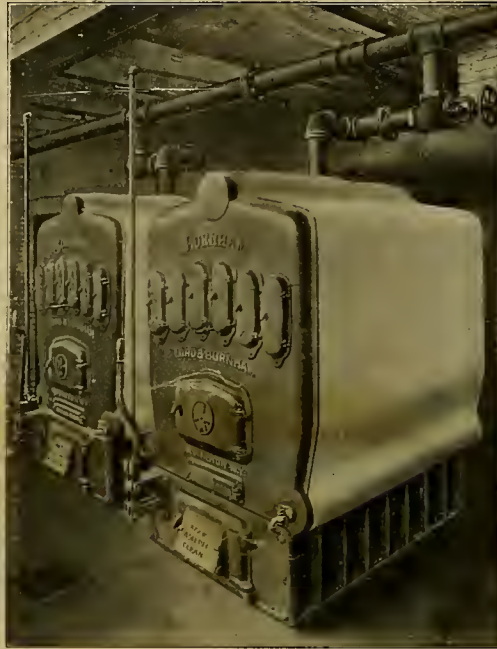
Get it out of your mind that setting boilers in battery requires complicated piping. This battery of two replaced one large tubular boiler in a greenhouse at Allegheny, Pa.
