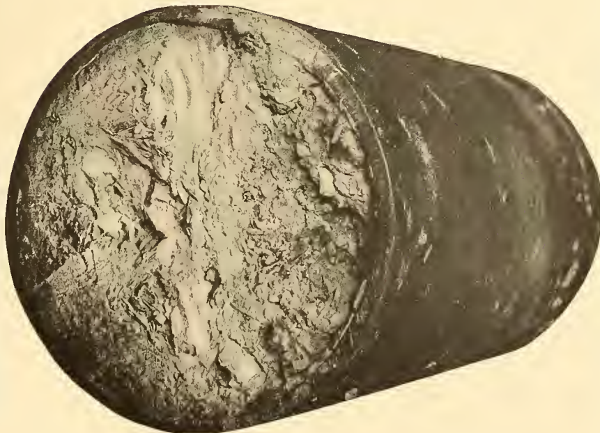
Fig. 1. Section of a boiler tube entirely closed with scale, taken from a neglected boiler in the provinces.
