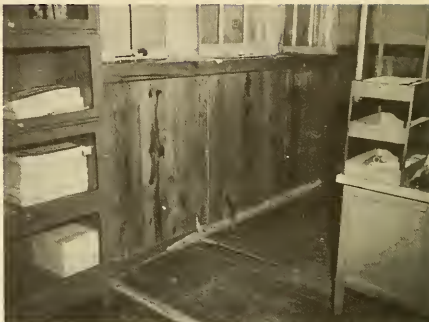
Damage to floor and base of cabinet
