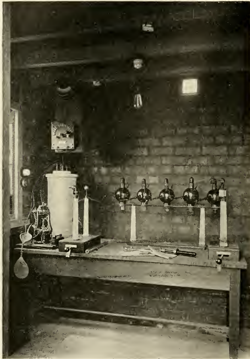
FIG. 108.—HIGH TENSION DISCHARGE APPARATUS AT DUMFRIES.
