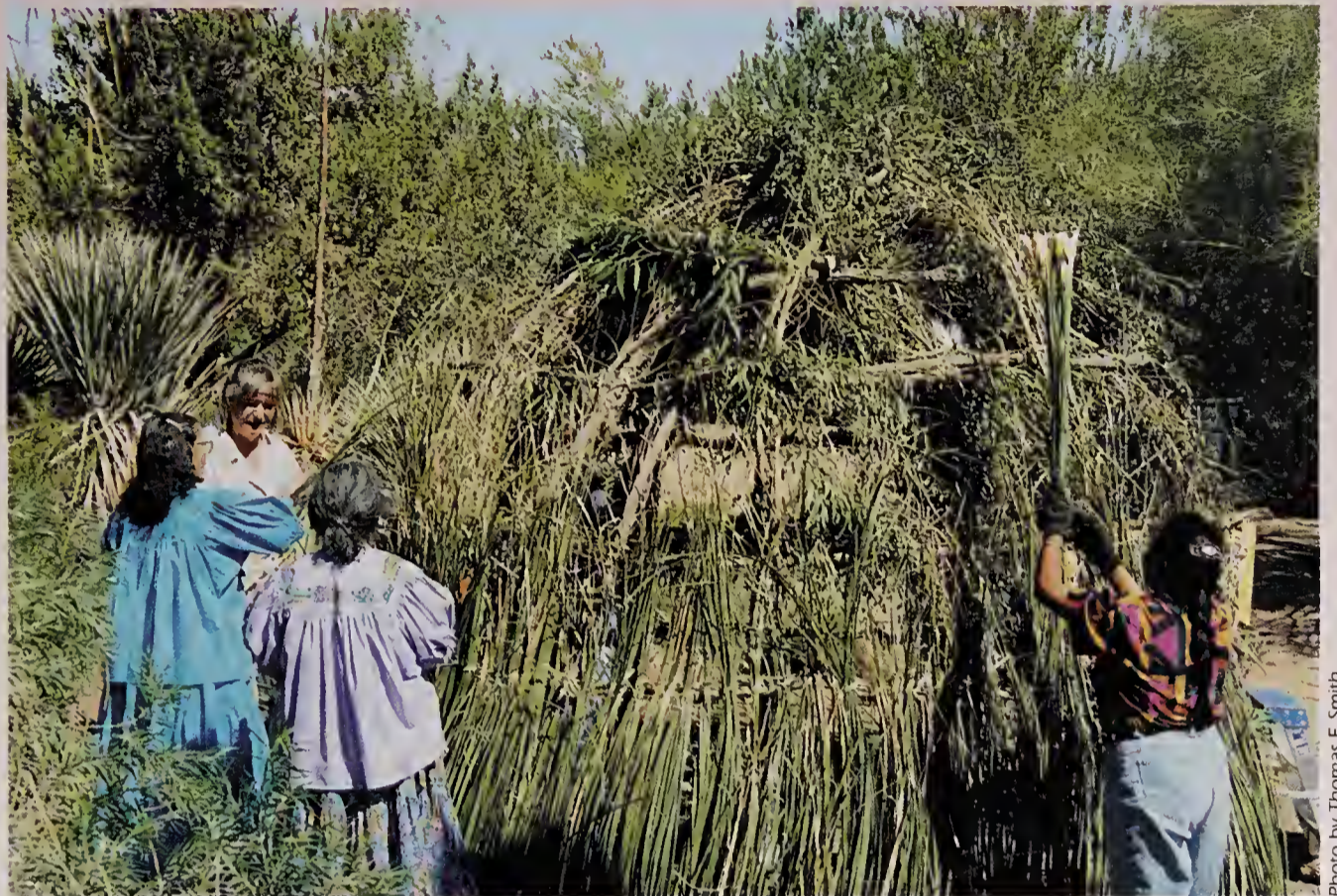
Apache women start to work on the beargrass installation on the exterior of a Wickiup.
