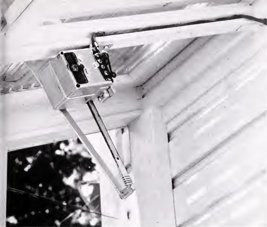
Motor for automatic control of greenhouse ventilators
