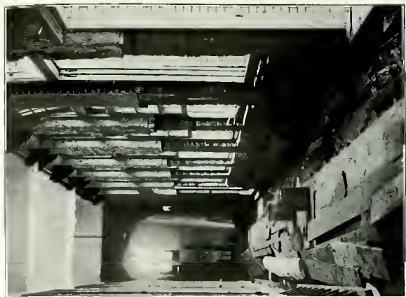
Fig. 2. Damage to woodwork on second floor of the building shown in fig. 1.
