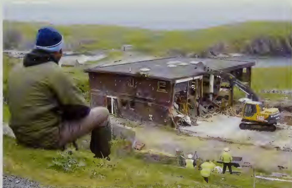
349. Fair Isle warden Deryk Shaw looks on as the remaining chunk of the old observatory, his home for ten years, was removed this summer. As we went to press, the site was clear and the foundations ready for the arrival of the new building, which is being put together in Orkney before being shipped to the island sometime this month. Thanks to those BB contributors who continue to donate their fees for photographs and text to the Obs Appeal www.fairislebirdobs.co.uk
